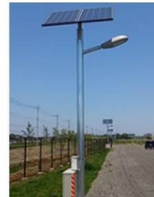
Solar panels installed at the Koga Plant 2.1 kw
